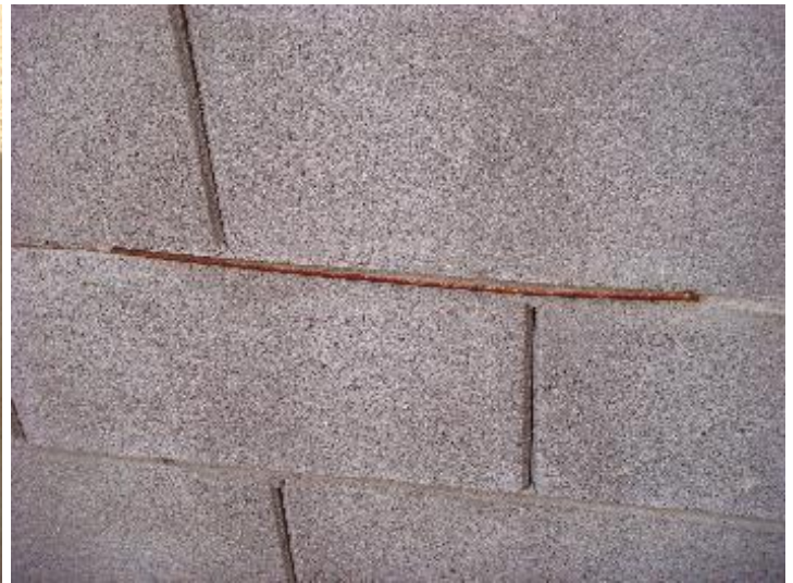
exposed metal on east wall
