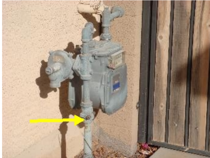
Gas meter was unlocked during inspection by gas company.
