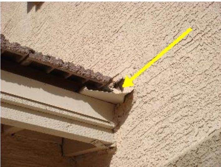
Damaged metal in kick-out
