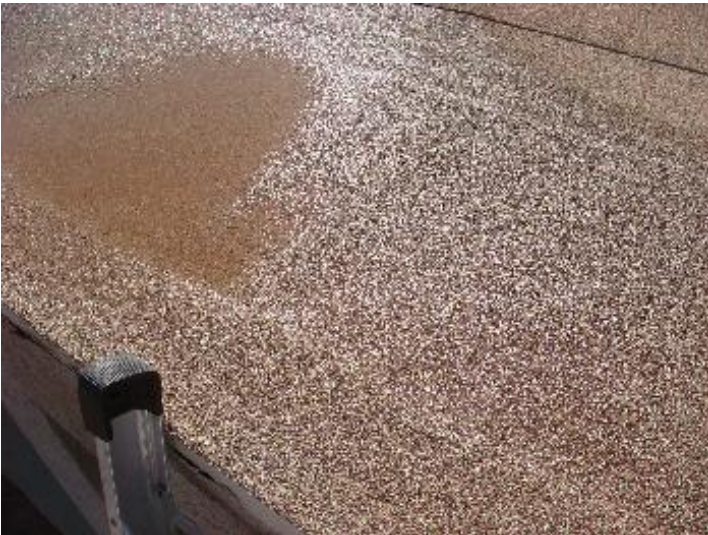
Ponding on patio roof
