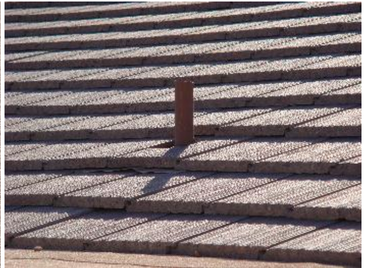
unusual vent penetration through tile
