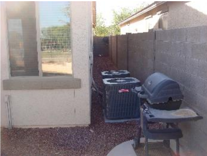
A/C units not level
