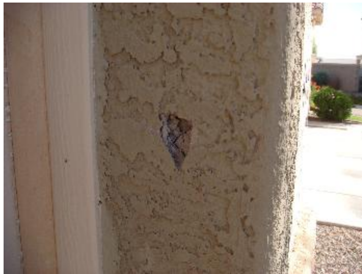
Hole in stucco with wire lath exposed
