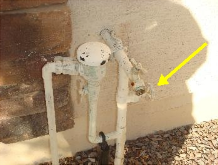
Main water shutoff valve
