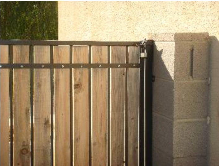
Exterior Fence Condition
