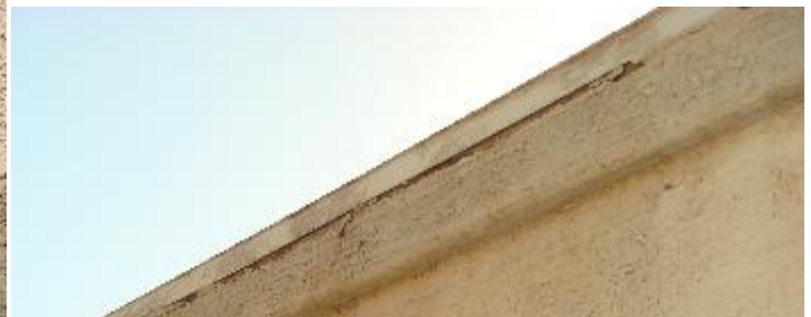
Stucco damage at drip edge on patio roof
