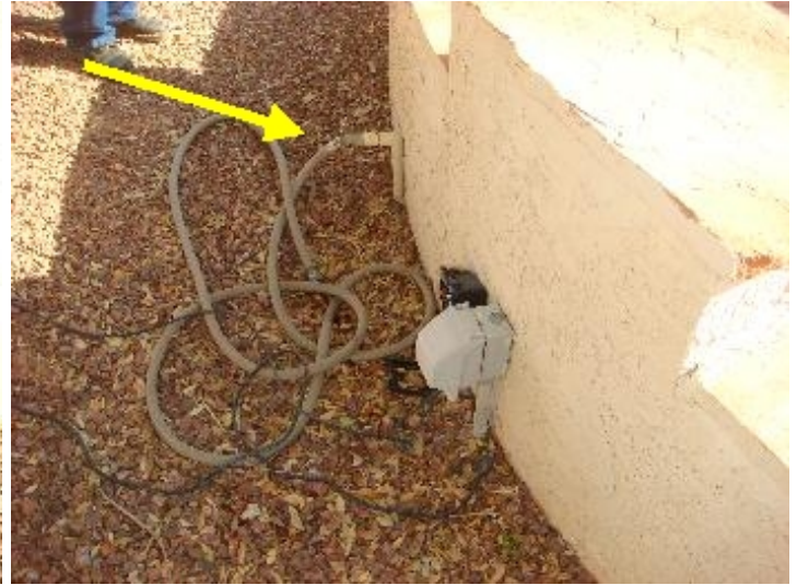
No anti-siphon on hose bib.
