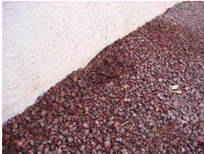
Extremely wet area with very soft ground
