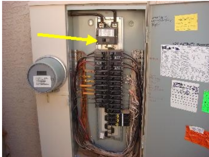
Service panel with cover removed. Main disconnect
